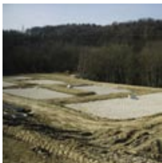
↑ Izgradnja rastlinske čistilne naprave s črpališčem za predčiščenje izcedne vode in vračanje na zasajeni del odlagališča Construction of constructed wetland with pump station for pre-treatment of leachate and recycling on planted parts of the landfill
