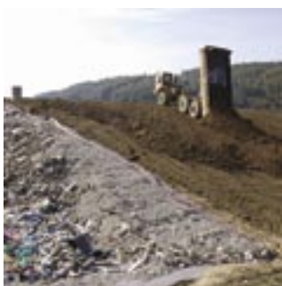
↑ Prekritje zapolnjenega odlagališča z zemeljskimi sloji in vgradnja podzemnega namakalnega sistema Covering of the filled landfill with soil layers and installation of underground irrigation system
